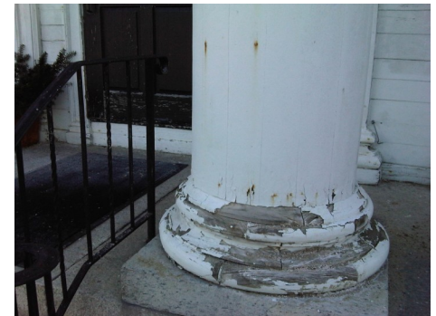
Crumbling column by front door
