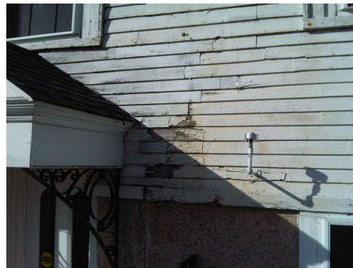
Peeling paint and water damage on south side
