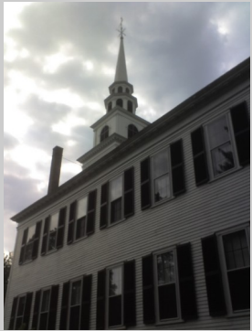
Peeling paint and rotting shutters
