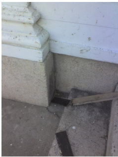
Pieces of crumbling shutters and peeling paint on east side by front doors
