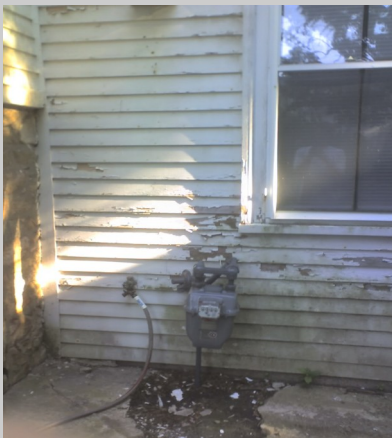
Peeling paint, rotting clapboards on north side
