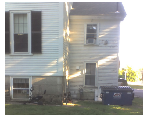
Peeling paint on northwest side
